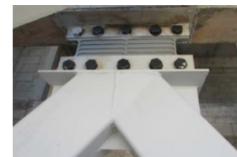
steel dampers (shear link device)
